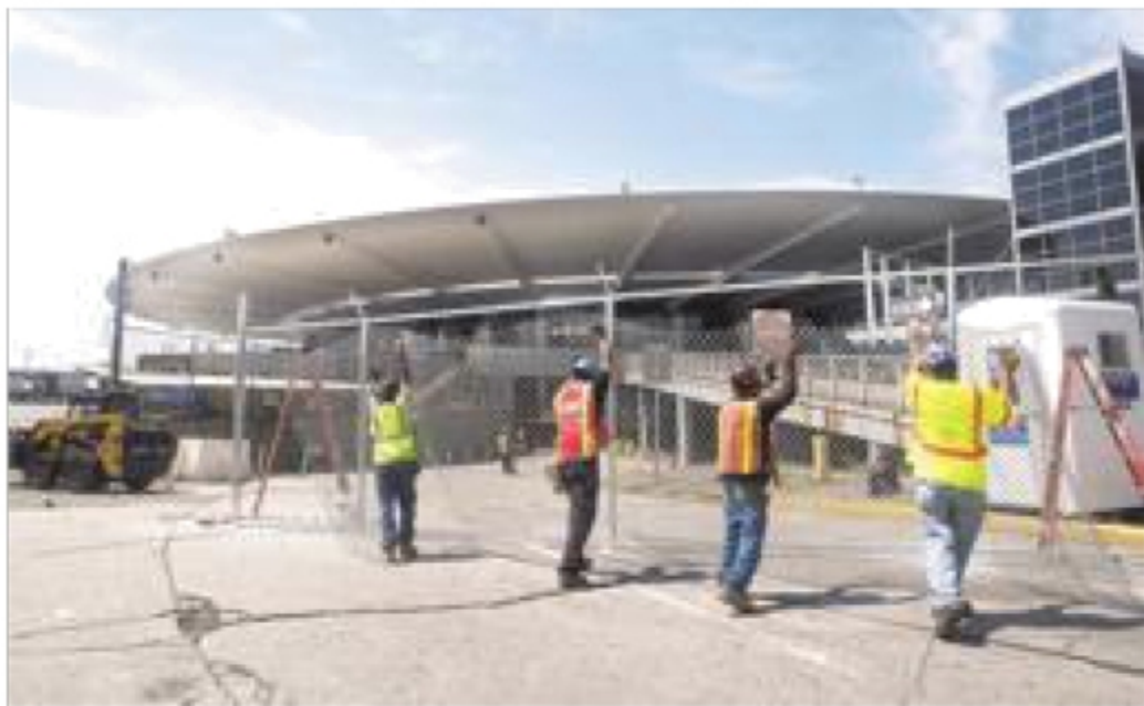
Construction workers set up a fence at the former Worldport Terminal at Kennedy Airport on Tuesday.
